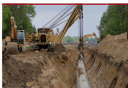
Bulk steel pipeline · Rand Water
