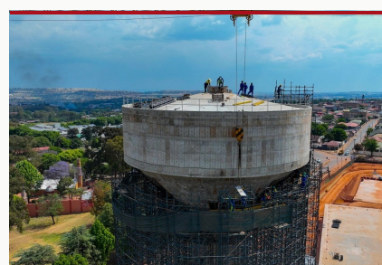
Brixton Tower & Reservoir
